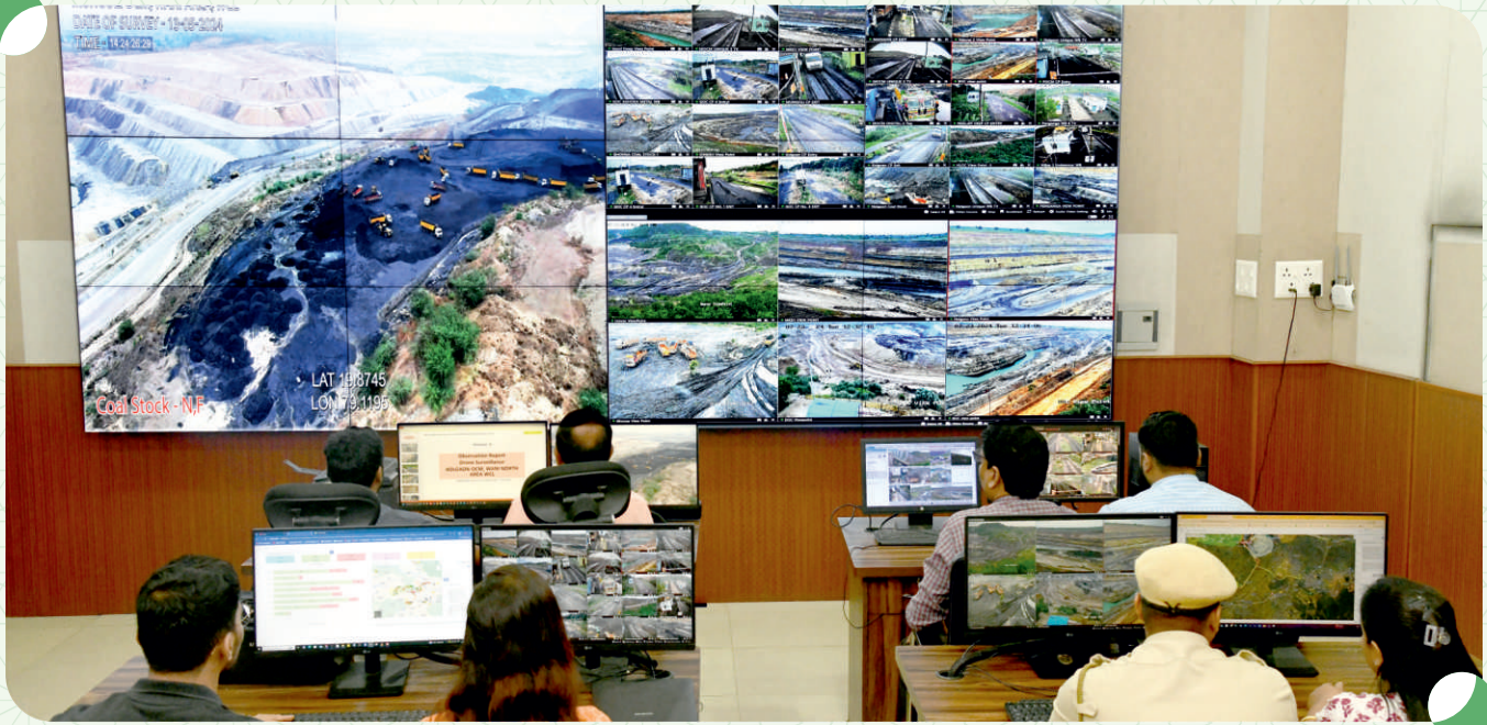
■ Integrated Command and Control Center (ICCC) at WCL HQ for e-Surveillance.
